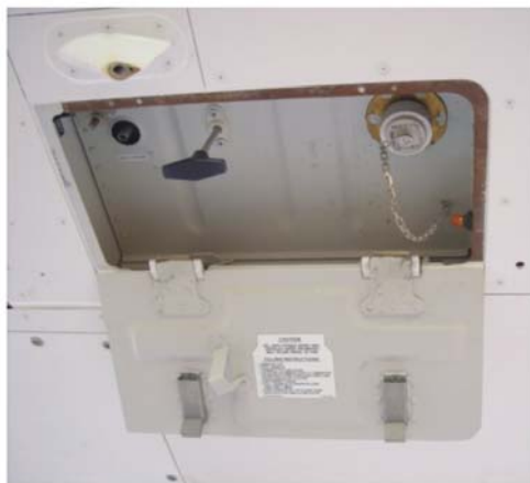
FIGURE 02-38-05-01 POTABLE WATER SERVICE PANEL DOOR AND TANK
